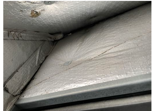
Photo 87- Rooftop Air Handler, Inside Fiberglass Insulation
