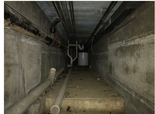
Photo 34- Basement, Southeast Tunnel, Fiberglass Insulated Hot Water Heater
