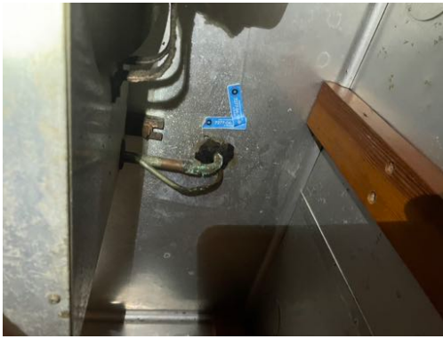
Photo 64- Sample #7277-04-16-04, 10% Chrysotile Asbestos Detected in Black Insulation Sealant
