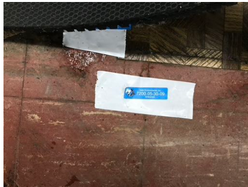
Photo 08- Sample# 7200-05-30-09, 5% Chrysotile Asbestos in Tan Floor Tile, <1% Chrysotile Asbestos in Black Mastic
