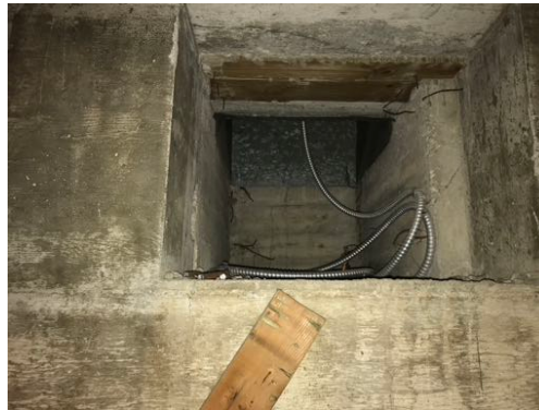
Photo 33- Basement, Southeast Tunnel, Uninsulated Ductwork
