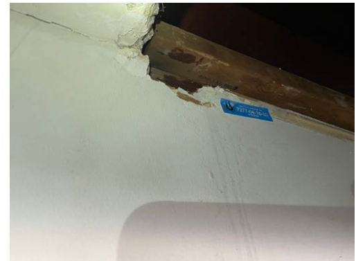
Photo 63- Sample #7277-04-16-03, 0.75% Asbestos in Joint Compound, No Asbestos Detected in Drywall
