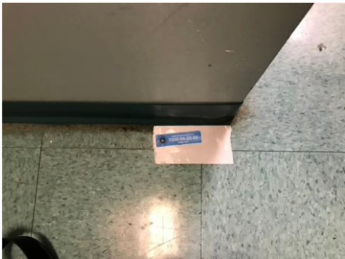
Photo 25- Sample# 7200-06-20-04, No Asbestos Detected in 12"x12" Aqua Floor Tile, <1% Asbestos in Black Mastic
