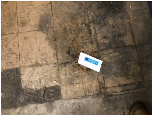
Photo 07- Sample# 7200-05-30-08, 5% Chrysotile Asbestos in Tan Floor Tile, 2% Chrysotile Asbestos in Black Mastic
