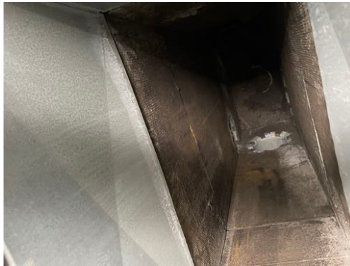
Photo 86- Rooftop Air Handler, Inside of Ductwork, Fiberglass Insulation, No Vibration Isolator Cloth
