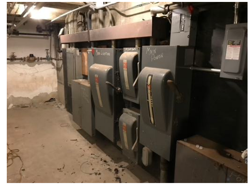
Photo 30- Basement, NE Hallway, North Wall, Central Area, All Electrical Insulators are Assumed to Contain Asbestos
