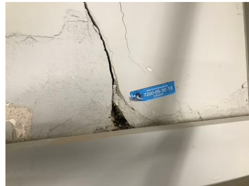
Photo 12- Sample# 7200-05-30-13, No Asbestos Detected in Hard Plaster on Wire Lath
