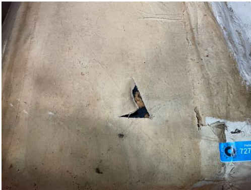
Photo 67- Sample #7277-04-16-07, 0.4% Chrysotile Asbestos Detected in White Sealant on Canvas
