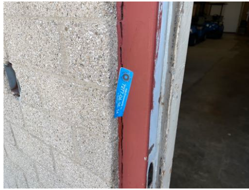
Photo 74- Sample #7277-04-16-14, 2.2% Chrysotile Asbestos Detected in Grey Exterior Caulk
