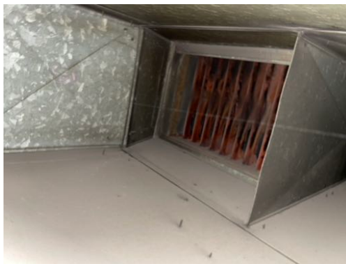
Photo 89- 1st Floor, Inside of NE Inactive HVAC Unit in Evidence Garage
